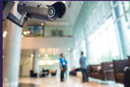
SECURITY EQUIPMENT & SAFETY
